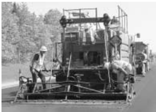
Microsurfacing on Interstate 75 in Michigan—one of 14 pavement preservation techniques in FHWA’s program.
