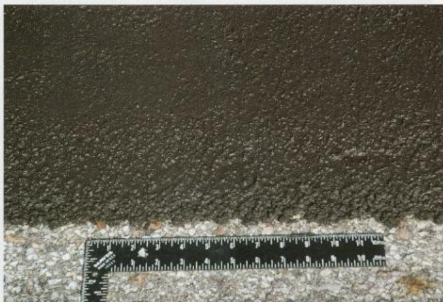
The microsurfacing asphalt emulsion—supplied by Jebro Inc. of Sioux City, Iowa—includes Butonal NX 4190 polymer, an emulsifier, water and, in the largest portion, PG 64-22 liquid asphalt binder. Photo courtesy of BASF Corp.
